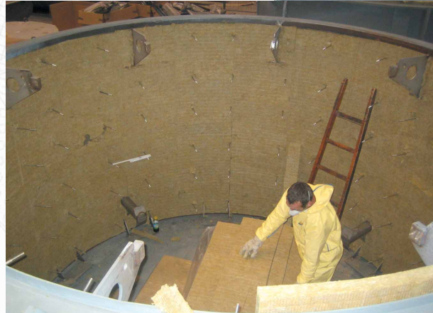
Work on the insulating of a shaft furnace. Rear insulating with mineral wool.
