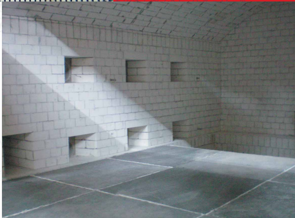
Complete refractory lining of a gas heated hearth furnace produced in refractory brickwork. Top of the furnace as vaulted ceiling (arched slab). Hearth plate made with refractory concrete.
