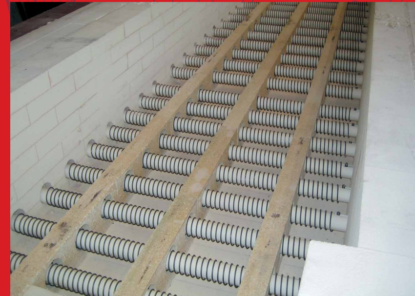
Heating system of muffle furnace. Heating spirals supported by ceramic tubes. Chamotte slab used for support. Side wall in refractory fire brick work.
